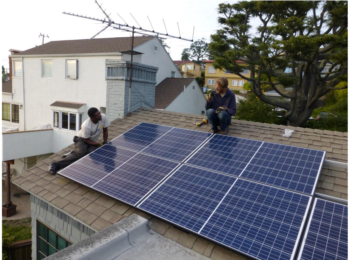
Courtesy Sunwork Renewable Energy Projects
